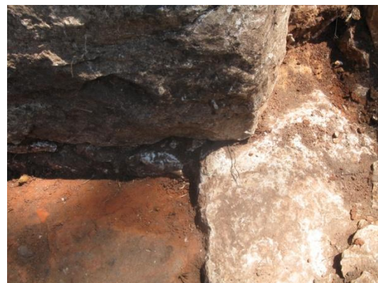
Detail of the northeast inside corner of the building under the corner of a large limestone boulder
